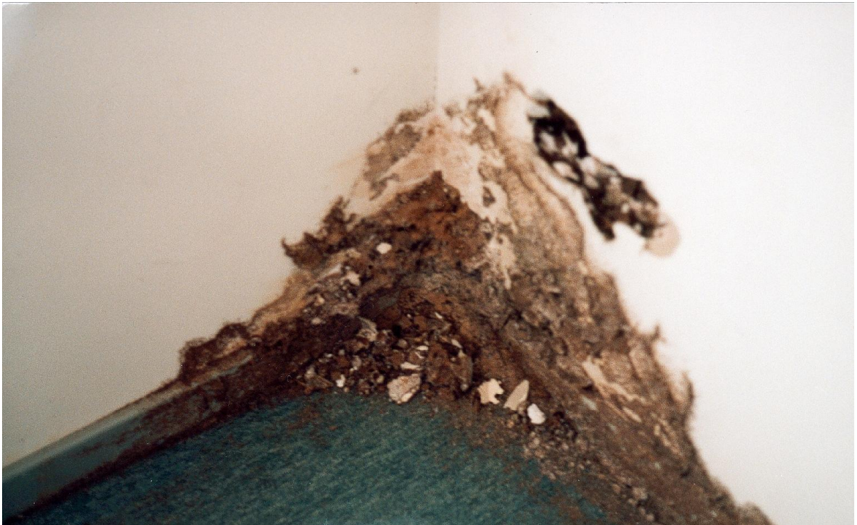
Figure 1 Southeast corner wall of main bedroom (where the daughter slept).
